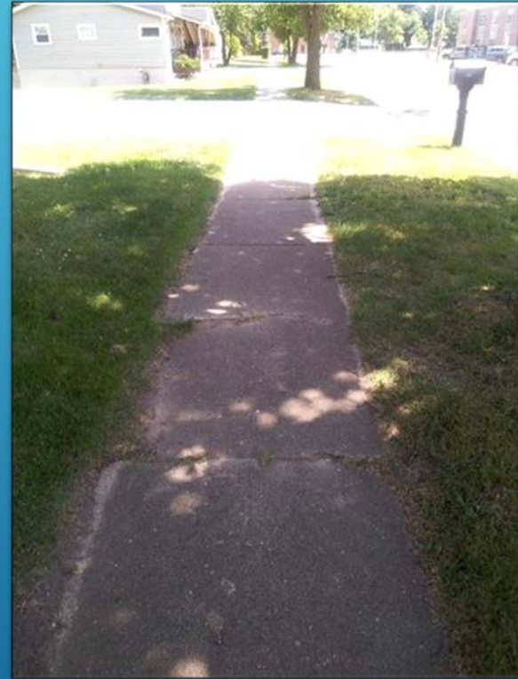
Settling on the sidewalk in front of 335 West Grand St
