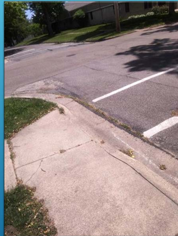
Non-ADA compliant crossing at South Jefferson St and West Bond St
