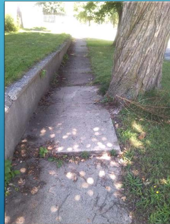
Sidewalk Uplifting in front of 501 North Boltwood St
