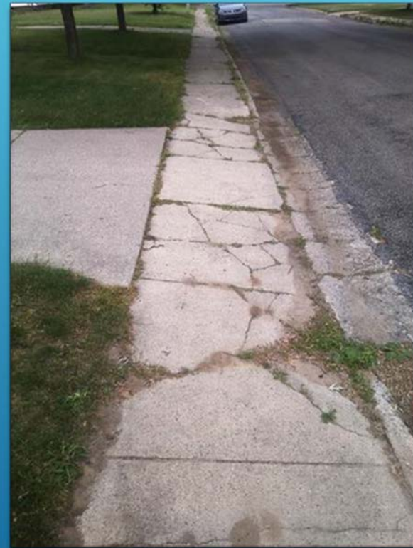
Cracking on the sidewalk in front of 620 W Madison St
